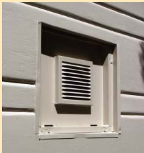
Figure 7. The house was too close to the property line for the author to install this heater outside, so he put it in an accessible crawlspace (top), ran the flue into a joist bay, elbowed 90 degrees, and vented through a grille in the outside wall (above).
